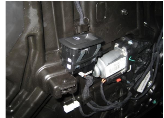
Neatly wire tie door switch onto the inner door panel so it does not protrude out past the other door parts.
